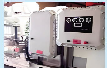
Zone 2 (Class 1 Division 2) Generator set package
