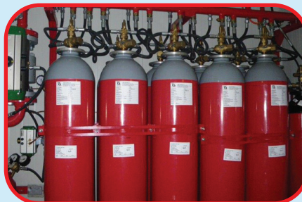
CO2 Fire Suppression System
